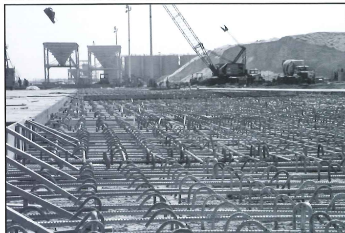
Coastal Steel employees installed this rebar for Berth 8 deck at Port Newark.
