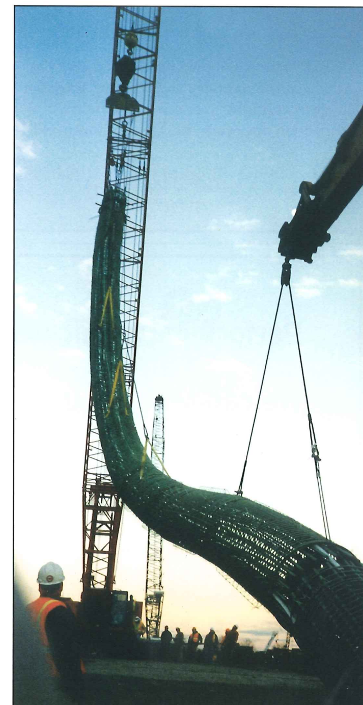
This rebar cage, constructed by Coastal Steel, is raised by a crane.
