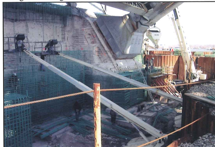
Coastal Steel Construction personnel installed this rebar on a Bayonne Bridge project.
