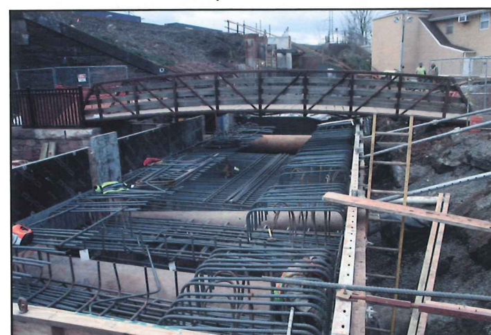
Rebar installed prior to concrete pour for a Green Brook Flood gate.
