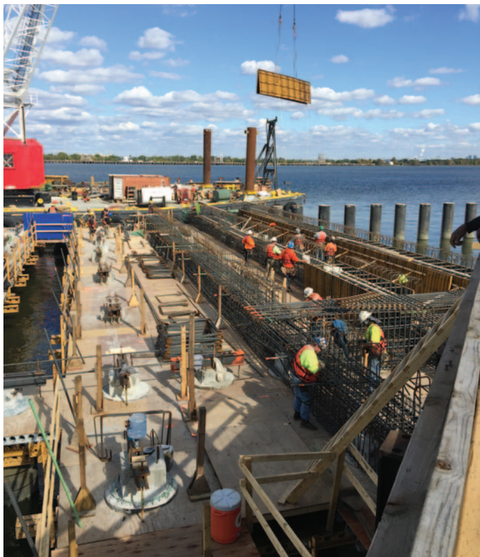
Paulsboro Marine Terminal Wharf (5,200 tons rebar) Phase I – Weeks Marine Phase II – Commerce Construction
