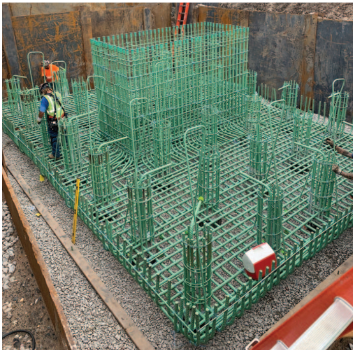
Newark Airport Terminal A Redevelopment Bridges N61, N62 & N63 (1,520 tons) Future AirTrain Foundation
