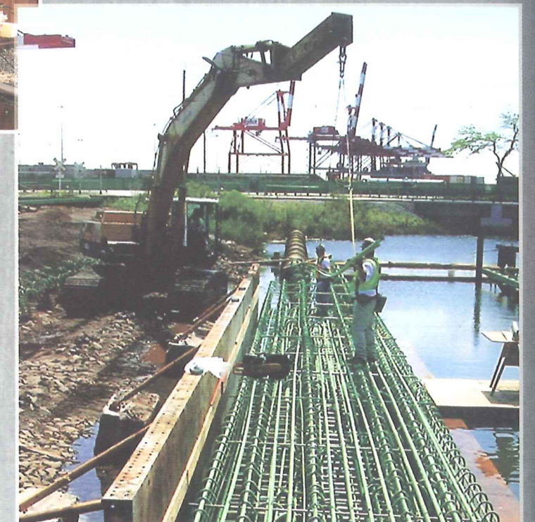
Construction of bridges for the intermodal rail support facility at Port Newark and Port Elizabeth.
