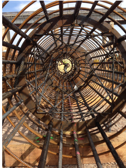
Coastal Steel Construction is producing caisson cages such as this to allow for underwater construction on the Goethals Bridge Replacement Project.
